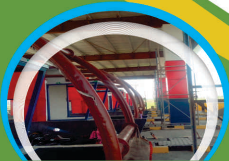
Toll booth protection frame:
